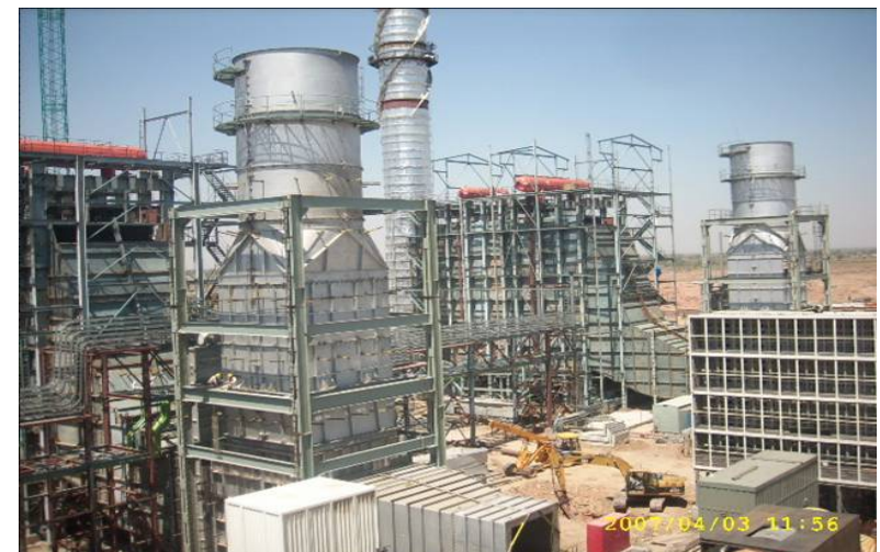
330 MW CCPP - RRVUNL, Dholpur, Rajasthan
