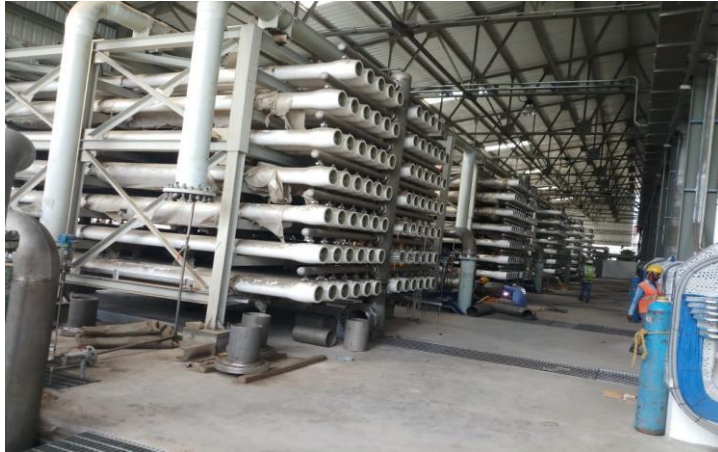
55 MLD Desalination Plant, AP
