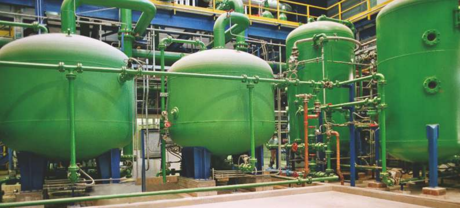
CPU Plant, 2x550MW Rutenberg Power Station, Israel
