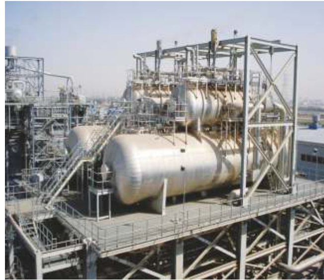
Deaerators at Jubail Water & Power Company, Al-Jubail, KSA
