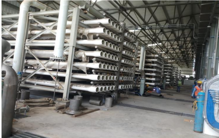
55 MLD Desalination Plant, AP
